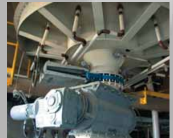
Cone and outlet of the multi-cell silo.
